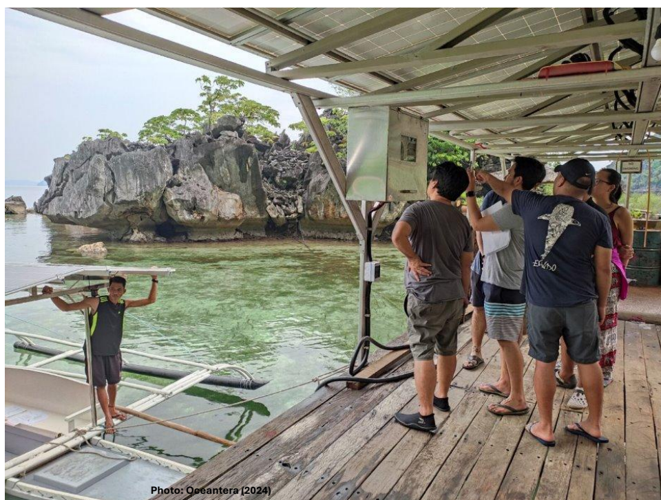
Figure 7. Charging station for Oceantera's e-boats.
